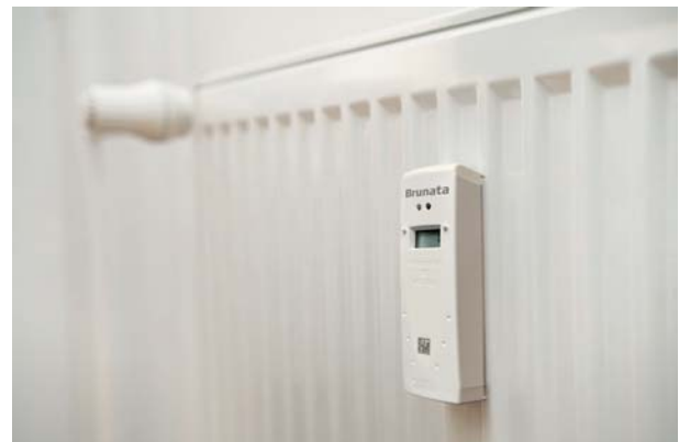
Figure 5.2: Heat cost allocator mounted on radiators
