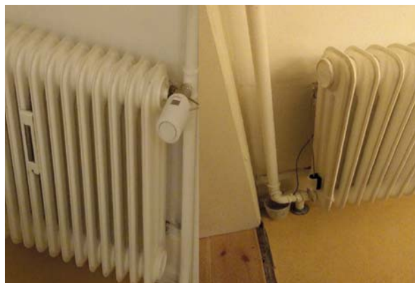
Figure 5.10: Example of the prototype thermostat and return temperature sensor and how they were installed on the supply (left) and on the side of the radiator (right) in the test buildings.
